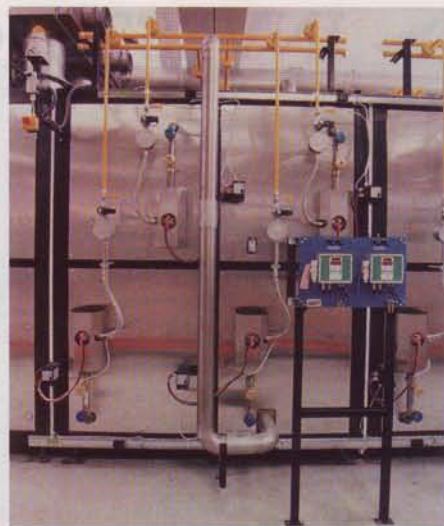
Burner heads on one side of the kiln, along with the related piping and the flow transmitters of the gas and combustion air.
