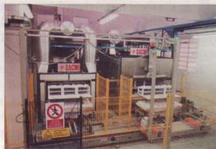
The kiln inlet (right) and the dryer outlet (left).
